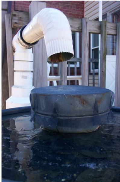
Figure 5: Screened Inlet to Rainbarrels
